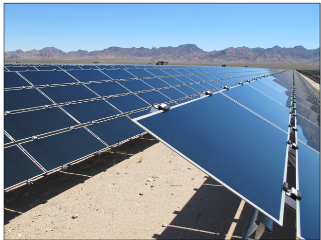
Silver State Solar, NV (BLM photo)
